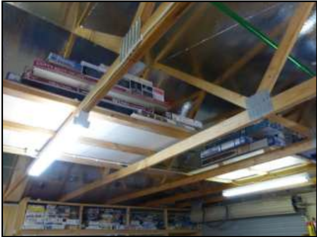
The stash and newly insulated ceiling to allow productivity during the summer months.
